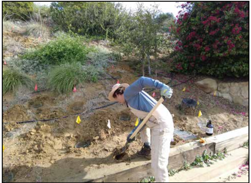
A CIR Field Technician hard at work on one of the restoration sites at Elings Park.
