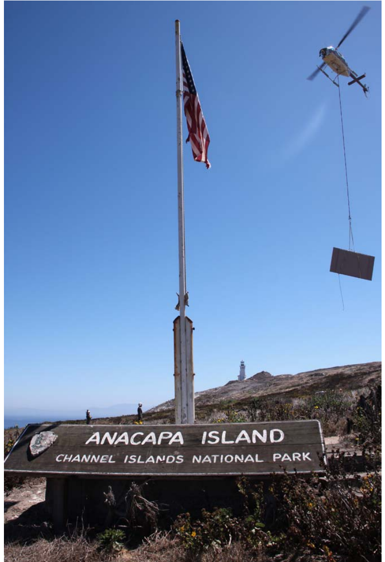
A helicopter delivers construction materials to the nursery site on Anacapa Island.
