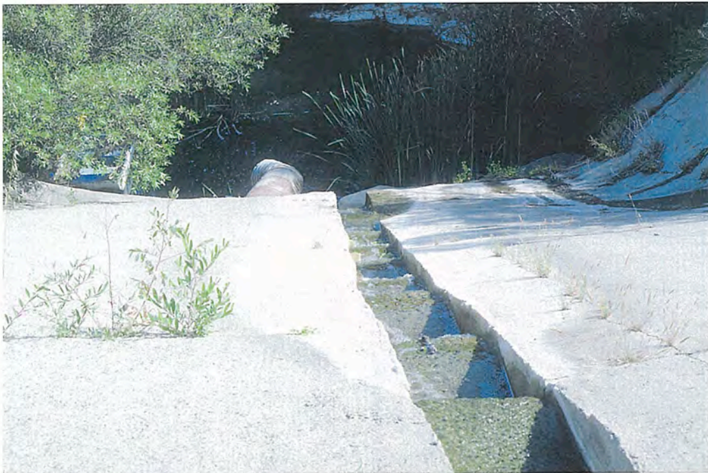
FIG. VII-8. SANTA BARBARA CO., HOLLISTER RANCH. View of a fish ladder, downstream from top of dam in a dissected coastal-plain canyon. Although the effort to provide access for fish to upstream habitats was well-intended, the small reservoir upstream from the dam has filled with sediment completely, resulting in a meadow-like plain without a clearly identifiable channel for use by fish.
