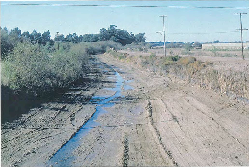
FIG. VII-7. SANTA BARBARA CO., GOLETA VALLEY, ATASCADERO CREEK. View downstream, westward along Atascadero Creek. The regional flood control district has maintained the flood capacity of such coastal plain streams by using bulldozers, backhoes, and dragline cranes to remove vegetation and sediment, thereby reducing the flood threat in urbanized areas. As shown here in 1983, all vegetation was removed except for willows on the left bank. In current practices, a preferred alternative that achieves riparian corridor management, including flood protection and preservation of wetland functions and values, has been implemented.
